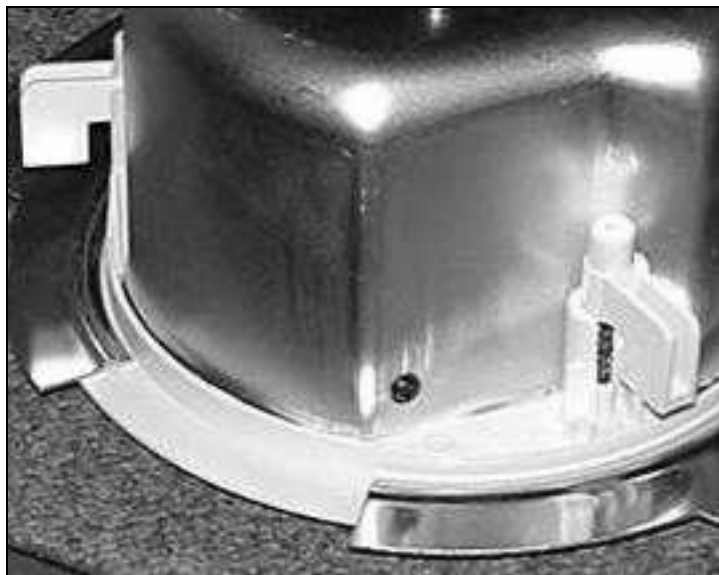
Loudspeaker in place.
